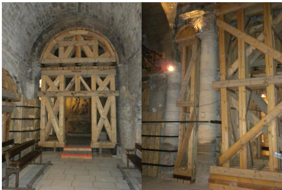
Figure 2. Examples of shorings – photos taken in the basement of the Saint Victor Abbey, in Marseille, France.
