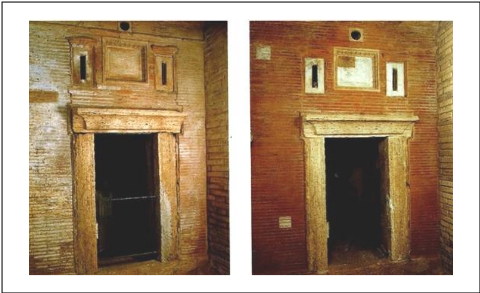
Figure 5. Vatican Necropolis, Mausoleum N, exterior south wall before and during the cleaning operation (from [3, p. 116], ©Fabbrica di San Pietro).
