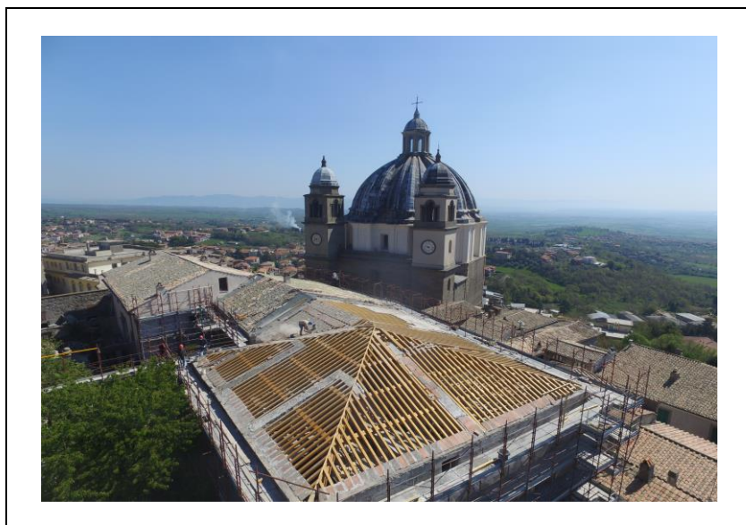
Figure 9. Restoration works of the Bishop Palace in Montefiascone by Andrea Gentili (6 th generation, 2016).
